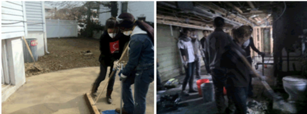
From left to right: cleaning up victim's backyard and removing basement floor damaged by seawater.
